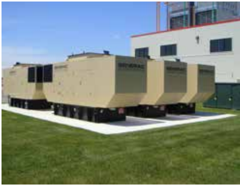
The Kenosha plant's mission critical power needs are solved by these five 600 kW MPS Bi-Fuel engines from Generac Power Systems
